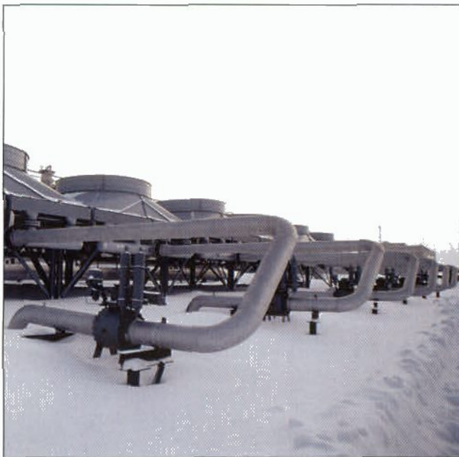
Figure 4.23 Natural gas processing in Russia Pictured here is a natural gas processing facility in Siberia, where the largest natural gas deposits in the world are located.
